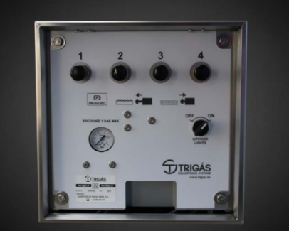
Pneumatic lift control panel
